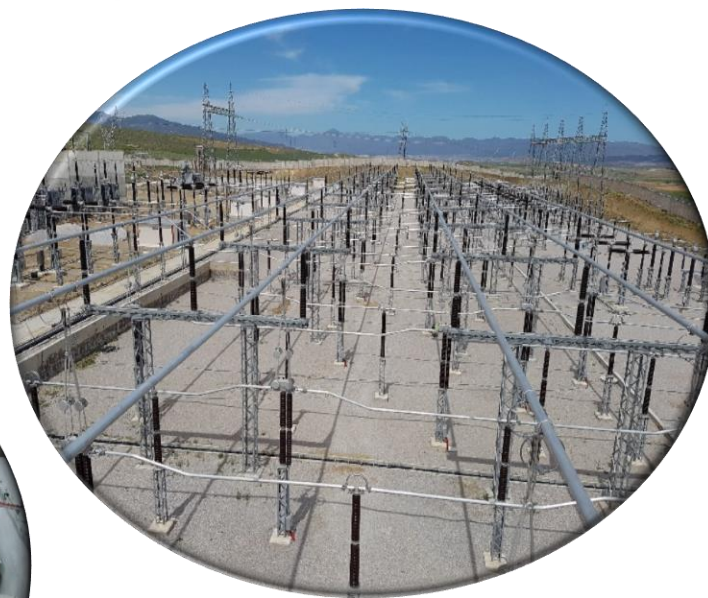
400/220 kV Tazoult Substation ALGERIA
