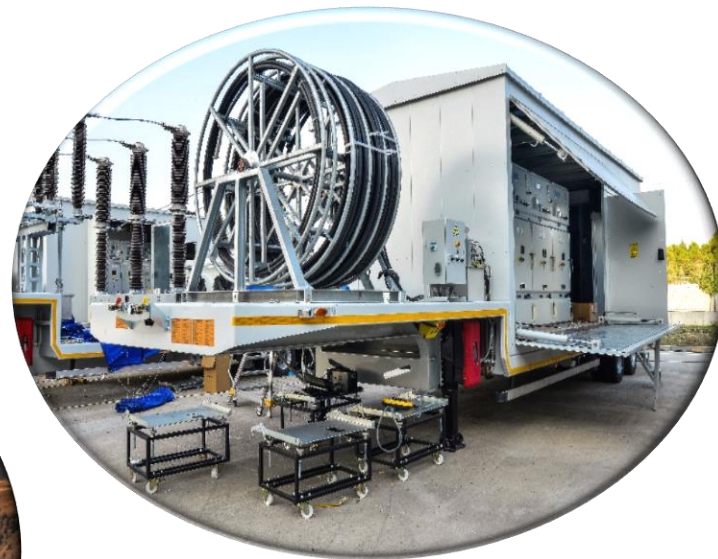
132/33/11 kV Mobile Substations IRAQ
