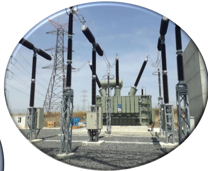
380/154 kV Çorlu Substation Extension TURKEY
