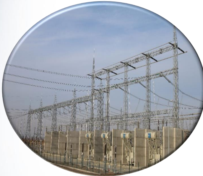
550kV Marnueli Substation GEORGIA
