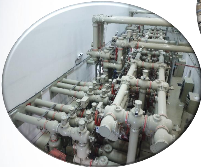
380 kV Bornova GIS Substation TURKEY
