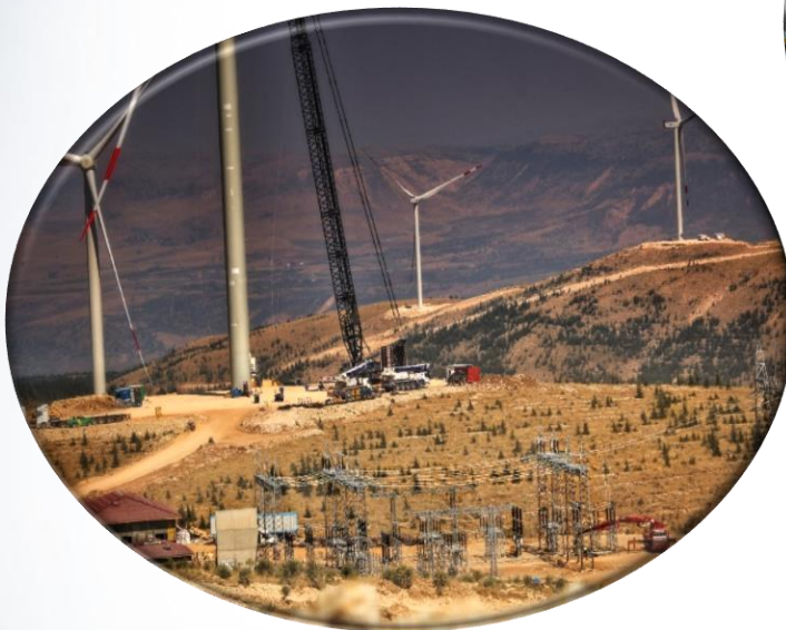
154 kV Cerit RES Substation TURKEY
