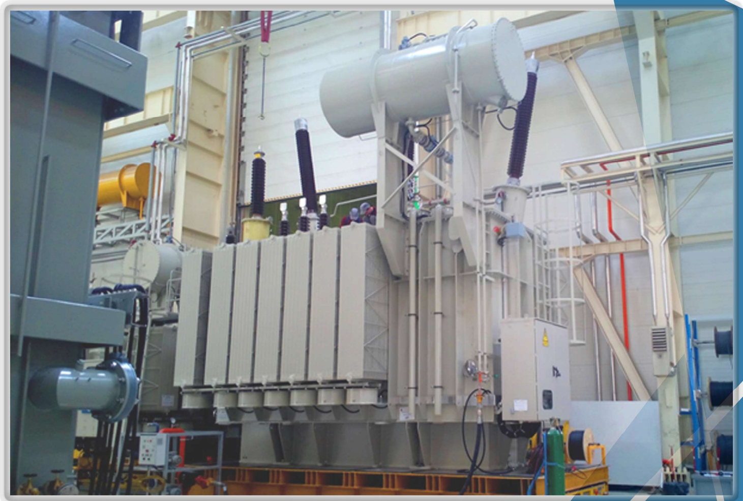
Pic. 1: SVC transformer before FAT
