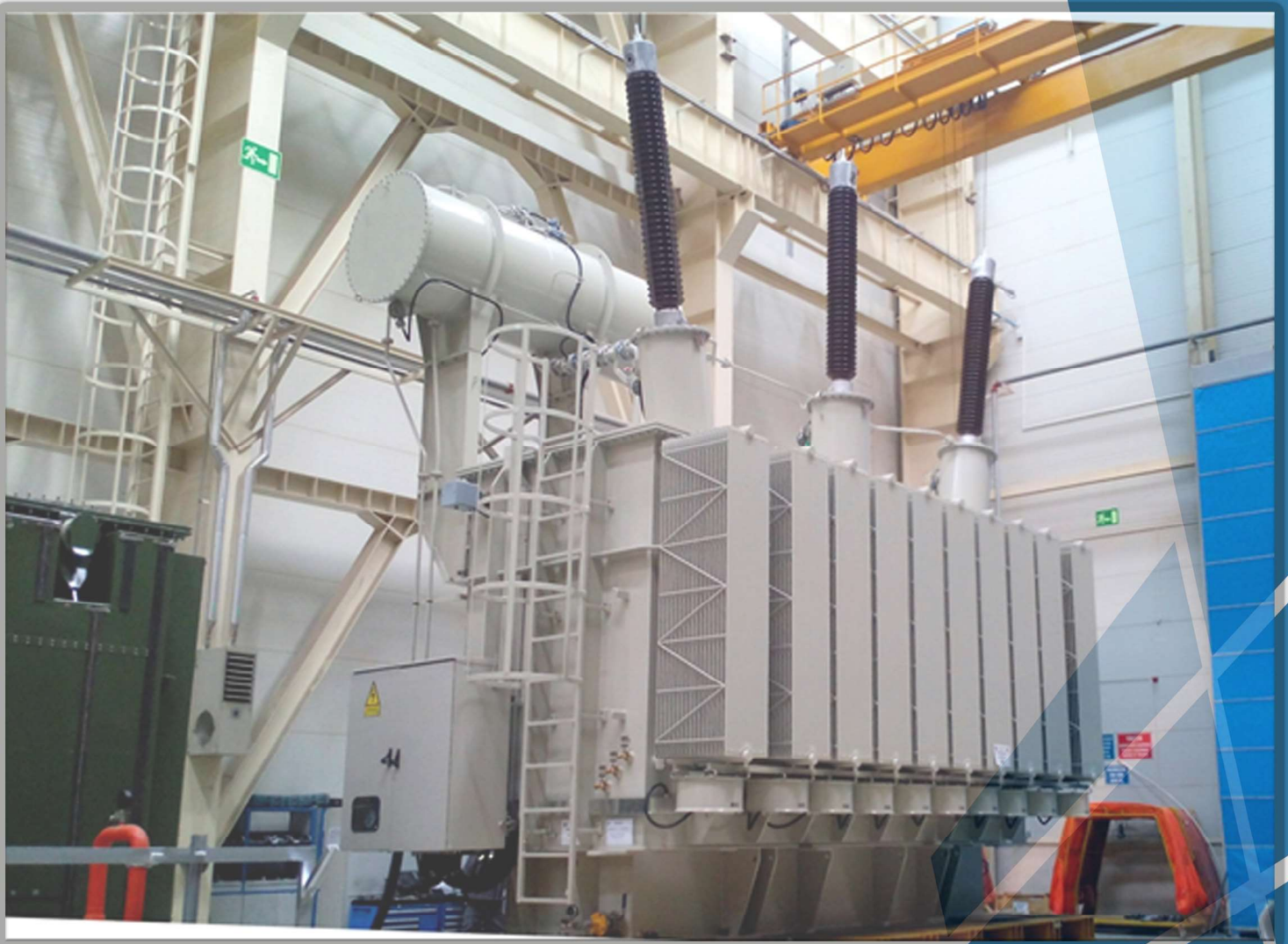
Pic. 2: Fully mounted SVC transformer
