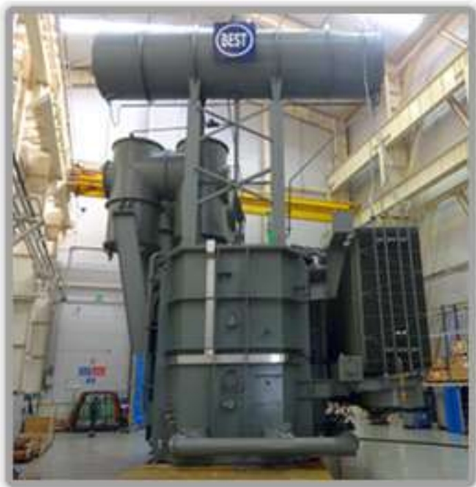
Pic. 2: 500MVA step-up transformer
