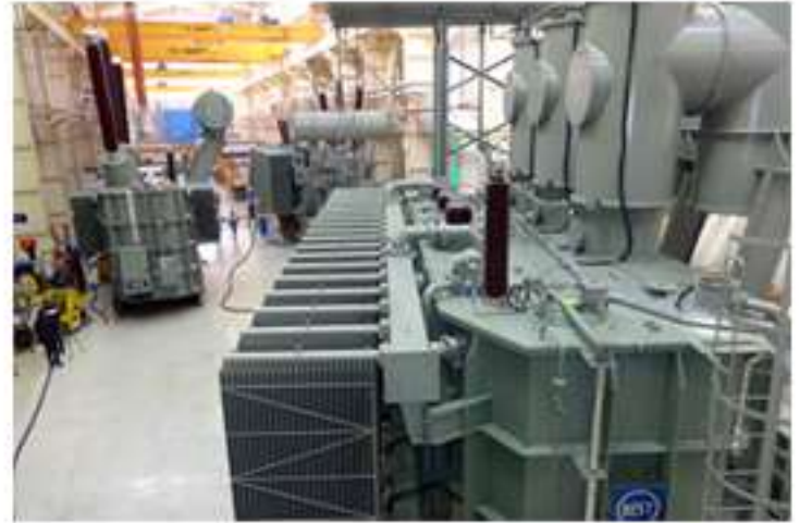
Pic. 3: Giant transformer is ready for test with all equipments.
