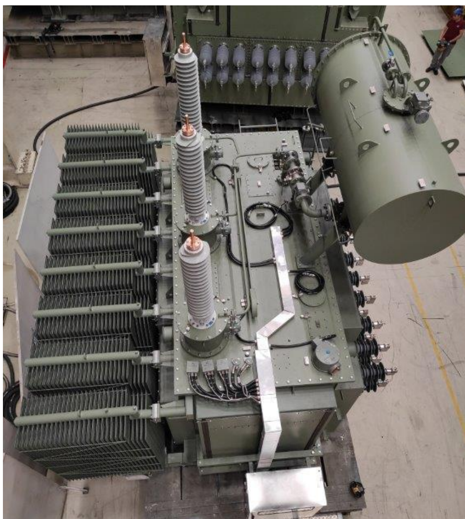
Figure 2: Converter transformer top view
