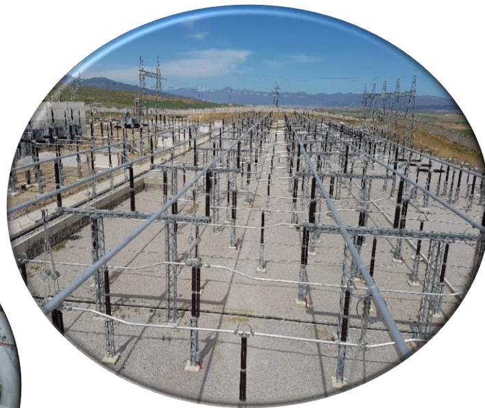
400/220 kV Tazoult Substation ALGERIA
