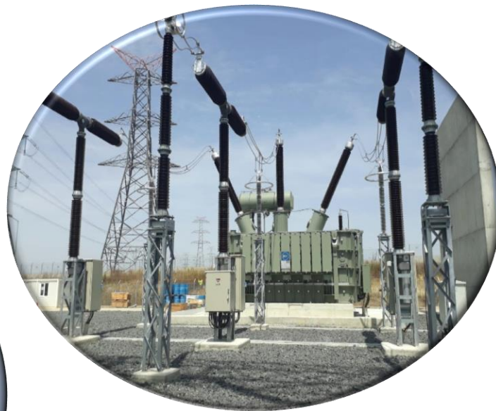
380/154 kV Çorlu Substation Extension TURKEY
