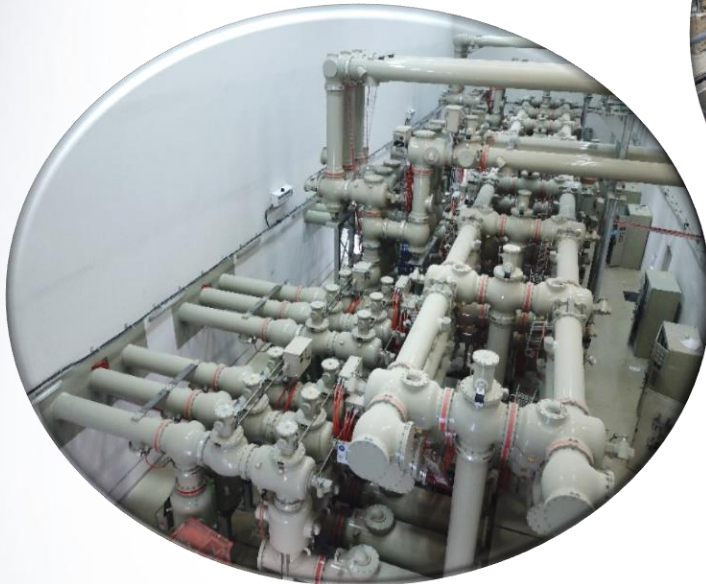
380 kV Bornova GIS Substation TURKEY
