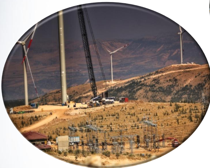
154 kV Cerit RES Substation TURKEY
