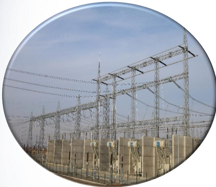
550kV Marnueli Substation GEORGIA
